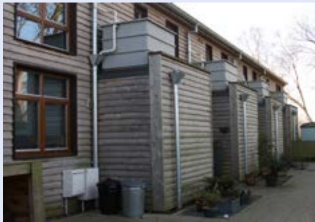
FIGURE 25: HOME RAINWATER CAPTURE SYSTEMS
